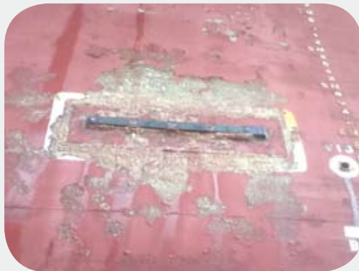
Di-electric shield in poor conditions
